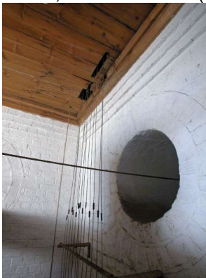
Above, is the second floor, ceiling, where the bell cables move upwards.
